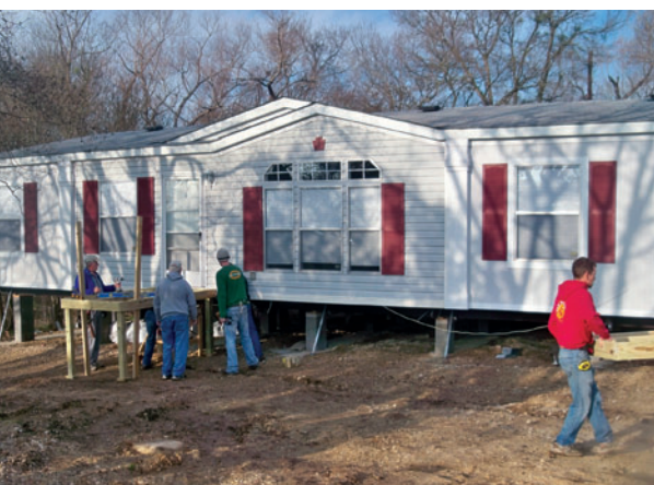
CTX partners with TX Ramp Project to help build two 60 ft. ramps to enable a disabled homeowner to access their mobile home
